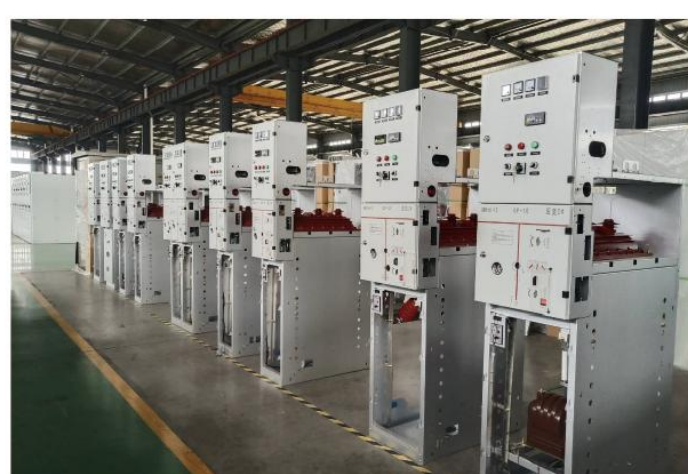
电力柜体 ELECTRICITY CABINET
